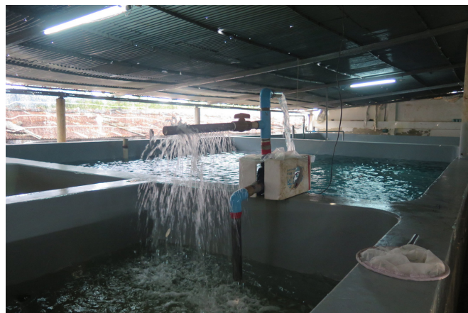
Figure 6: Water filtration and ingress
