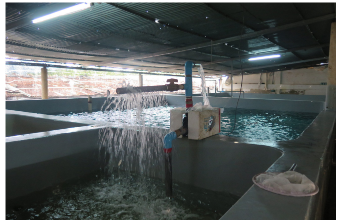
Figure 6: Water filtration and ingress
